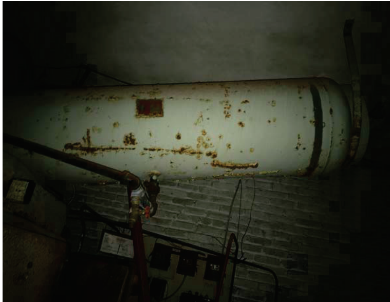
Photo 19: Boiler Tanks [Basement Boiler Room]
