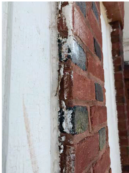
Photo 26: HA26 Exterior front door caulking (B74-B76) 5% Chrysotile
