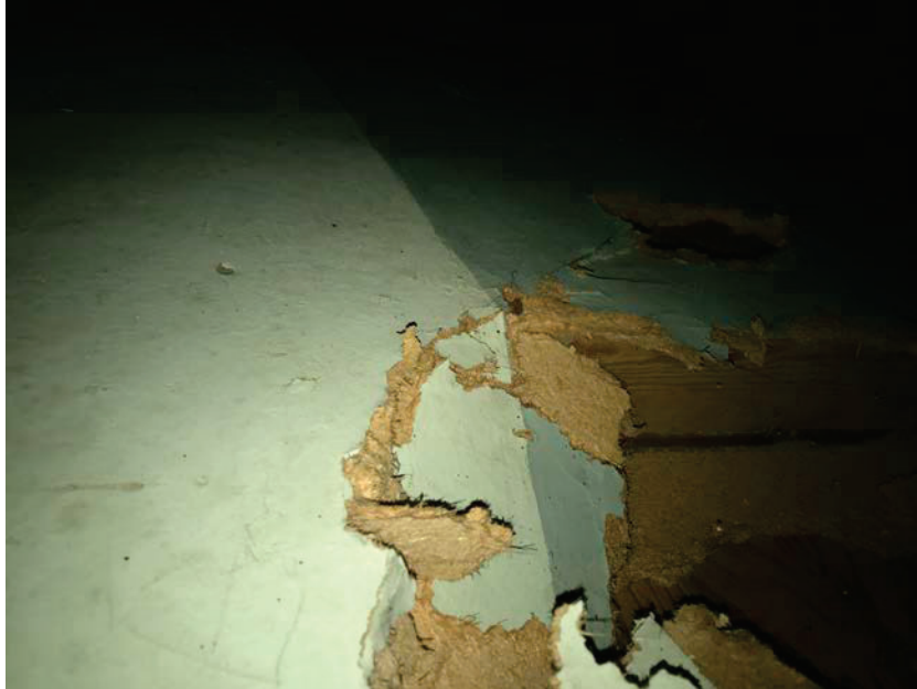
Photo 15: HA15 Brown drywall in basement classrooms (B42-B44)
