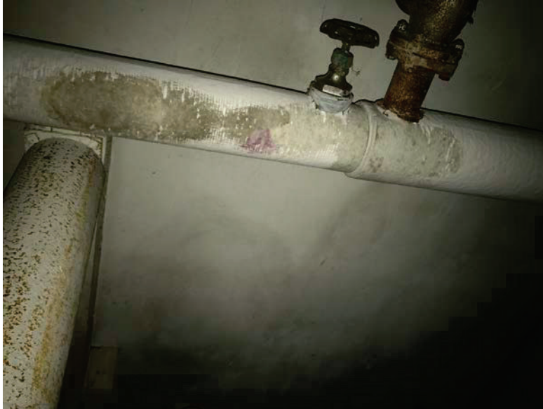
Photo 20: Boiler Pipe Insulation [Basement Boiler Room]
